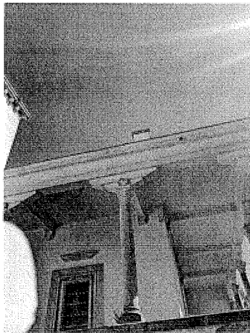
Streasina infiltrarea apei/ atac biologic
